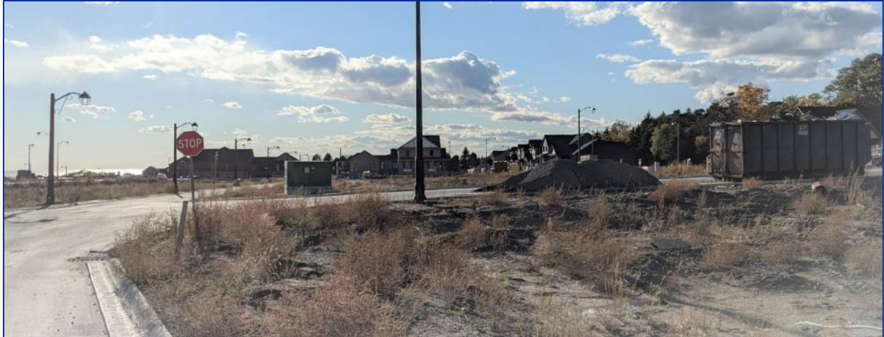
Figure 22: View west on Strachan Street of new residential development under construction along the north edge of the Study Area.
