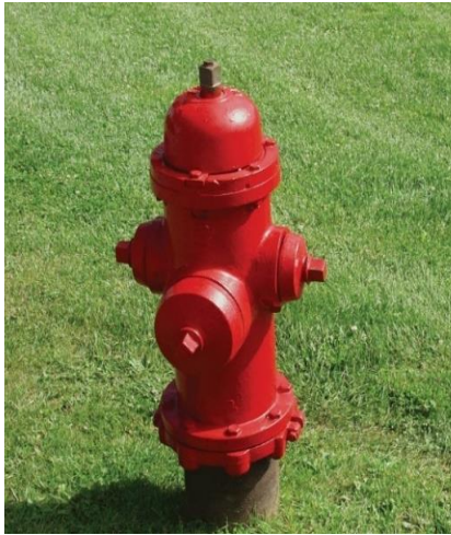
Figure 42: Picture of private hydrant.
