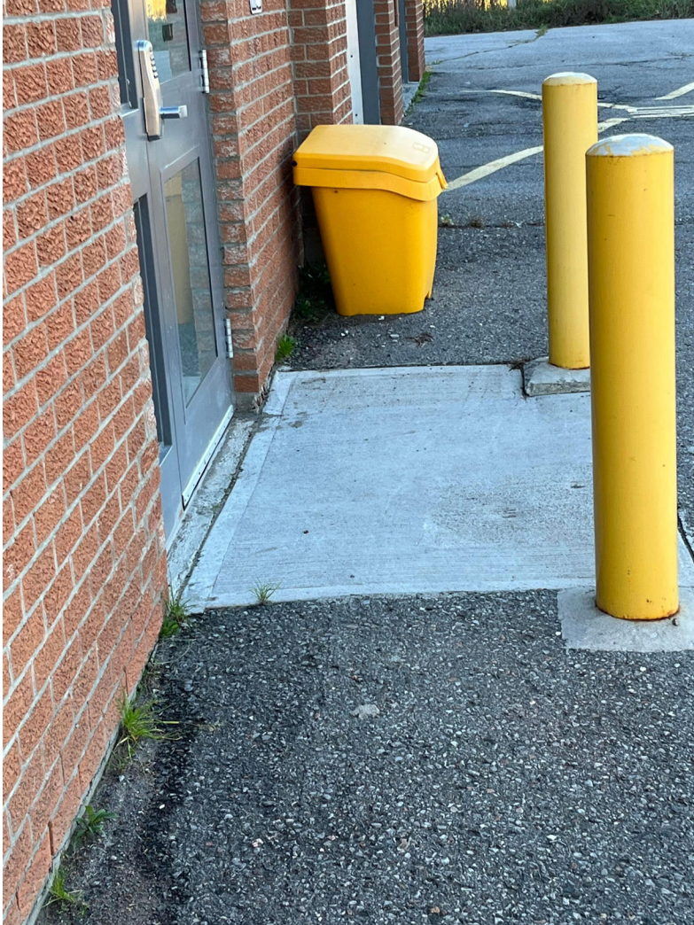
C:\Users\whitehead\Desktop\Fire Station 3 ( wrong grade on cemnt - Bunker Room door).jpg
