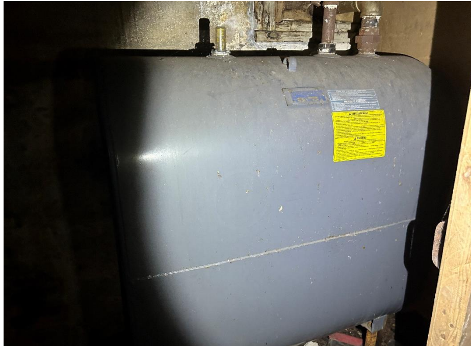
Photo 5 AST observed in the basement of Site Building B, September 28, 2023.
