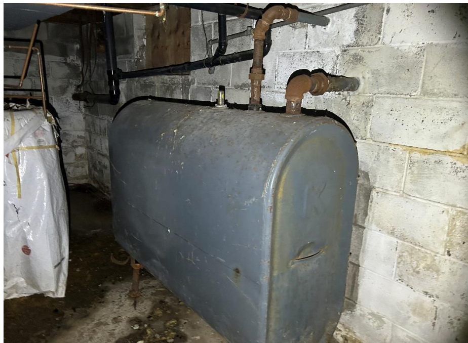
Photo 4 AST observed in the basement of Site Building A, September 28, 2023.
